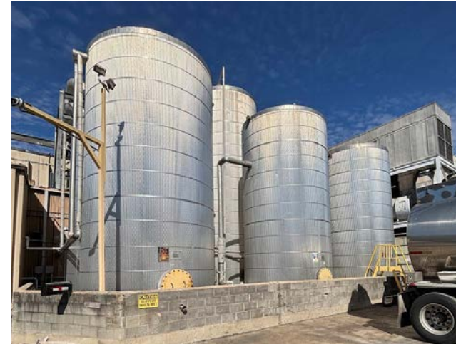
PVA Recovery at our Blacksburg, Textile Manufacturing plant (U.S.). PVA is recovered from wastewater and the water is reused for other textile operations.
